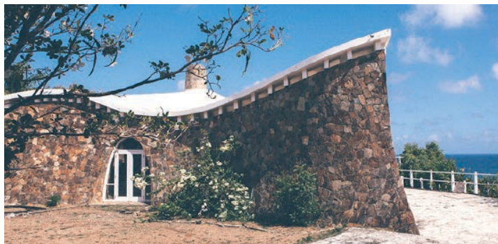
The northern façade of the building designed by architect Nelson W. Aldrich, its terrace with an unparalleled view over the bay of Colombier, and the interior. The house has been damaged over time, and hurricanes Luis and Irma accelerated its deterioration.
